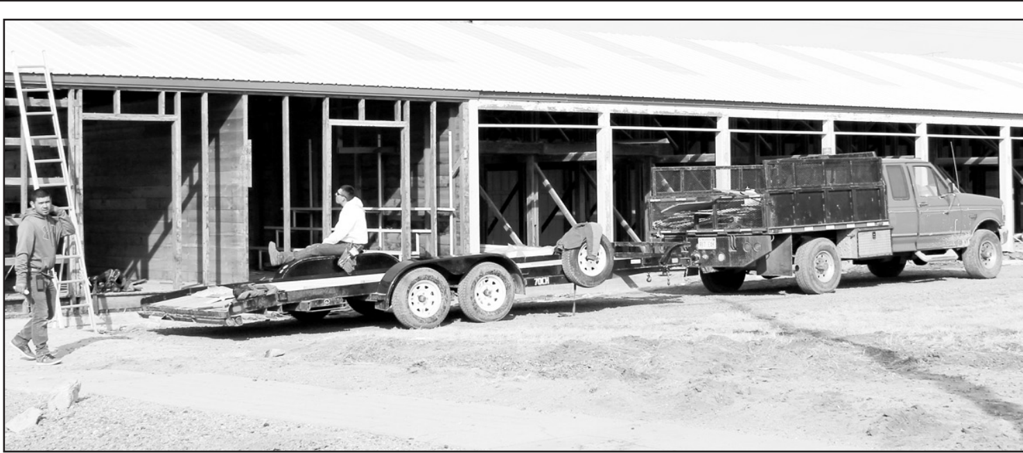
NEW BUSINESS in progress on East Fifth Avenue! Clint Bursch and Cliff Leach bought the old lumber yard, and are constructing storage units named Cougar Storage. Jose Cruz Davila and his crew with Vap Construction in Atwood, have been working to have it ready for an April opening. Times photo by Norma Martinez.
