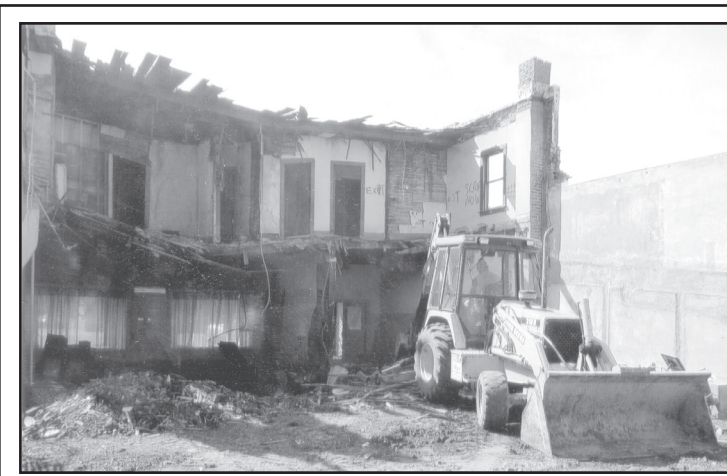
DEMOLITION has begun on the old Movie Theater that was condemned years ago. Work is being done by Roy Shrader. Times staff photo by Norma Martinez.
