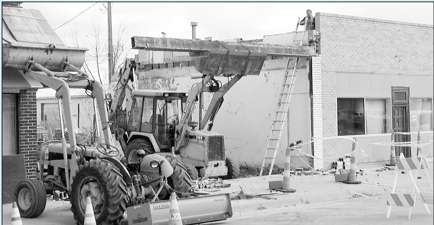
FINAL PIECES of the old theater building came down as Roy Shrader looks on.
