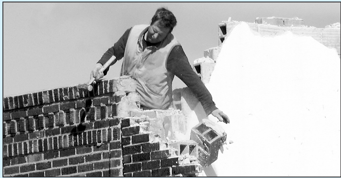
ROY SHRADER takes off pieces from the Senior Center, making sure the wall remains intact after the old theater building was removed.
