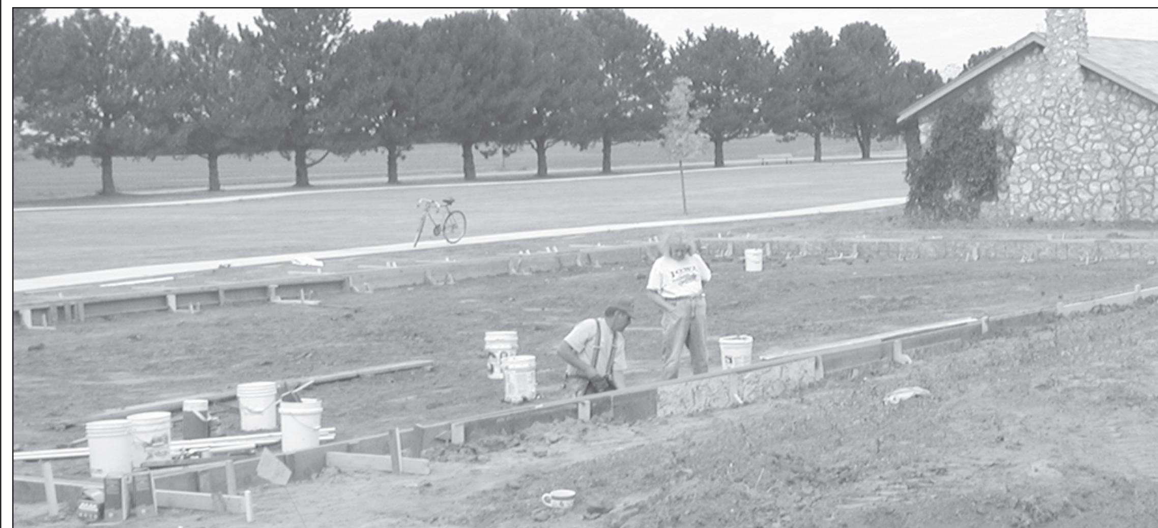
ROY SHRADER AND DAWN PETTY build forms to construct the new volleyball pits at the park. The sand for the new pits will be donated and will come from Benkelman. Times Staff photo by Melinda Basnett
