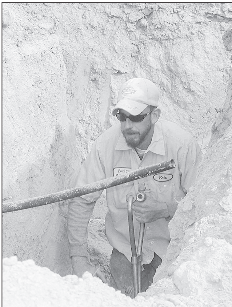
ERIC BARTELS, CITY MAINTENANCE, installing meter barrels at the Middle-Income Housing project on 5th Street.
