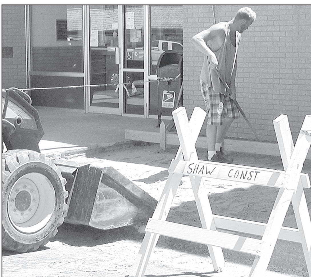
BEN SHAW with Shaw Construction, Benkelman, replaced the sidewalk in front of the Bird City Post Office. Times staff photo by Norma Martinez
