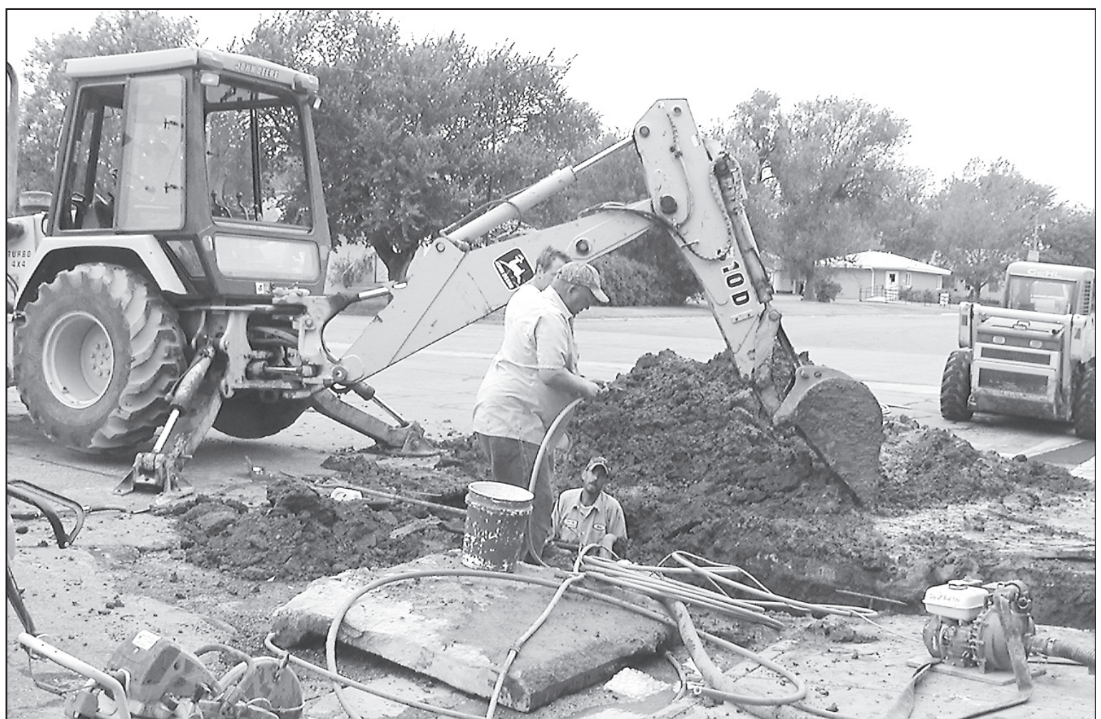
CITY WORKERS REPAIR pipes in front of the Senior Center. Pictured is Brad Schneider, city superintendent, Roy Shrader, local contractor, and Eric Bartels, city maintenance. Times staff photo by Norma Martinez.
