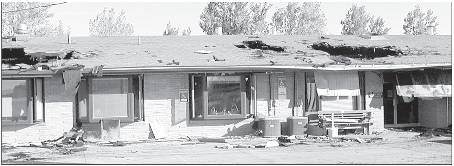
FIRE FIGHTERS made holes in the roof of the Good Samaritan to access the fire and get it under control.
