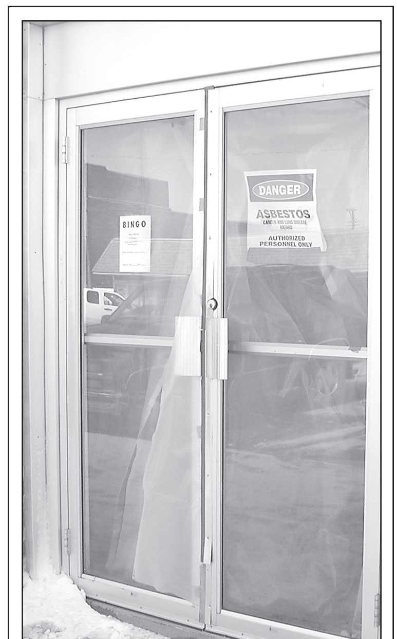
ASBESTOS tile is being removed from the Legion hall. Times staff photo by Norma Martinez
