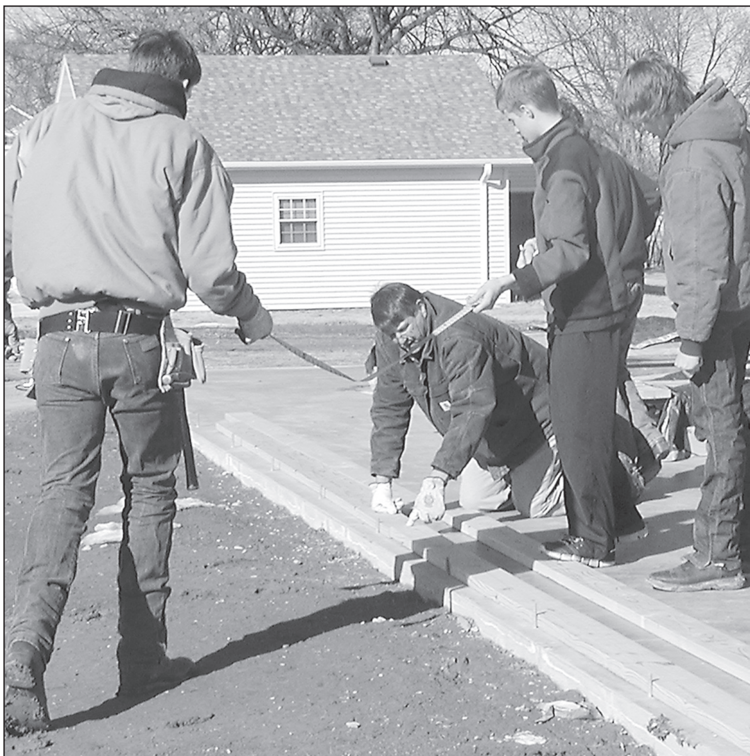
WELLNESS CENTER construction is underway. Students in Dennis Hengen's class are getting a lot of building experience. Pictured left to right are Josh Keltz, Dennis Hengen, Ty Carmichael and Connor Hazuka. Times staff photo by Tim Burr
