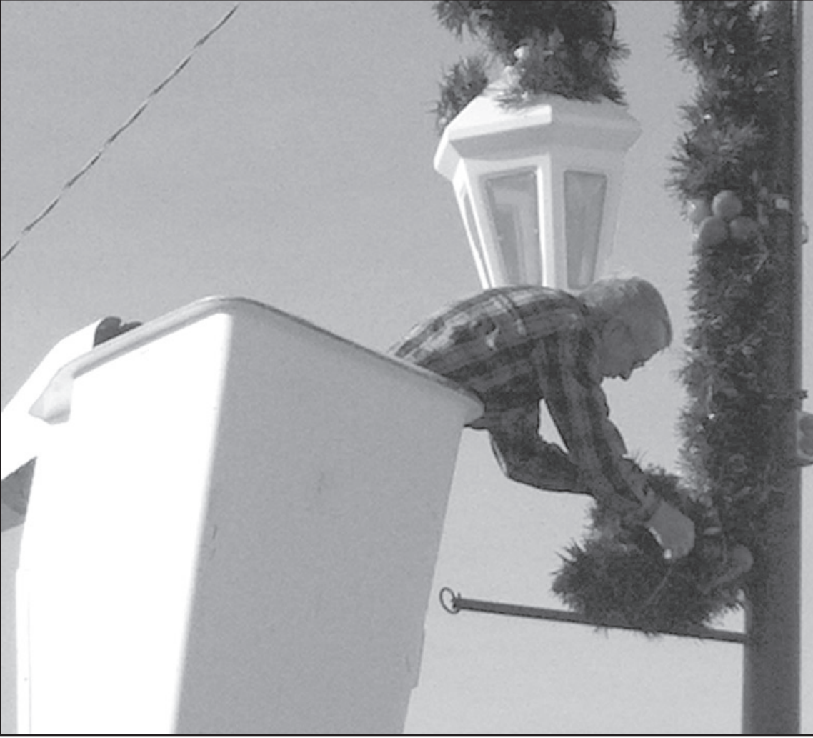
EVERY YEAR, the Wrights use their bucket truck to hang the Christmas decorations in Bird City. Above, Don Wright wraps garland around the pole.
