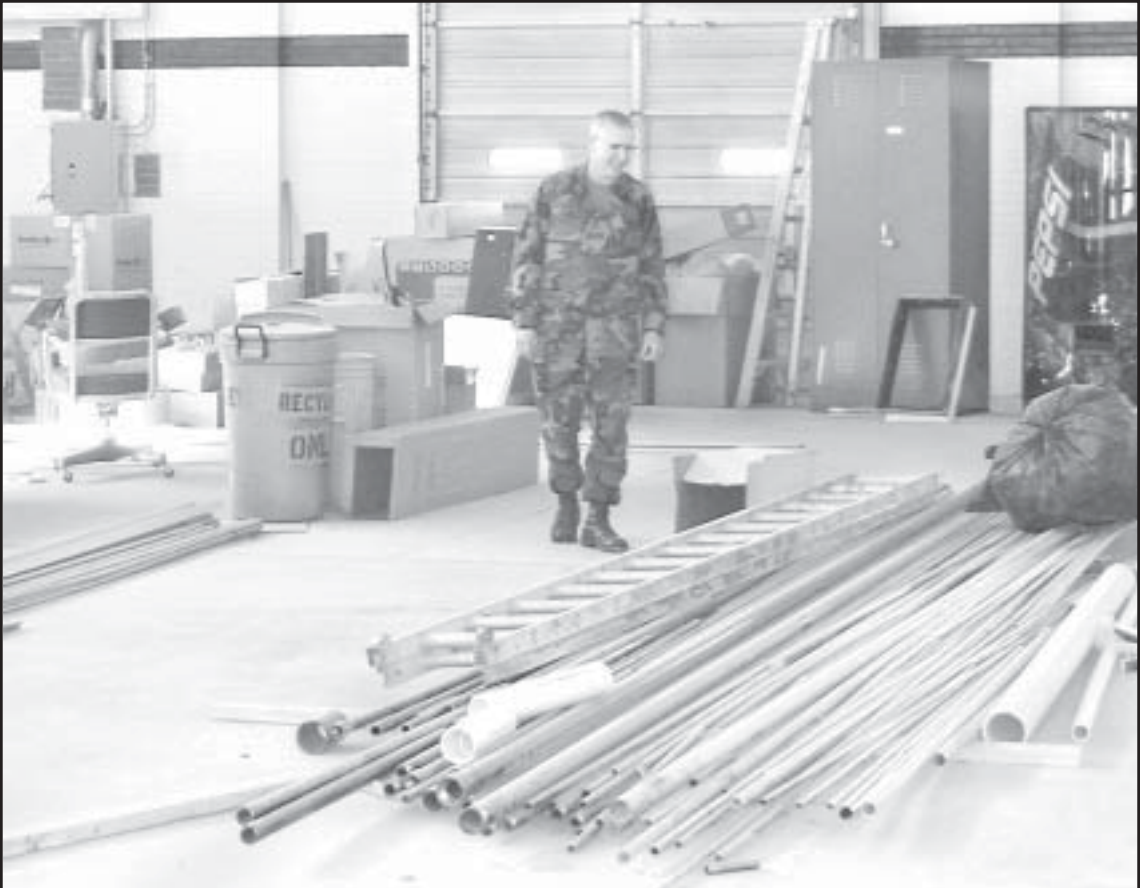
Staff Sgt. Bill Neff, walks around construction debris and materials layed out on the floor of the Norton National Guard Armory that is being refurbished. The project began in September and is expected to be completed by April. — Telegram photo by Carolyn Plotts
