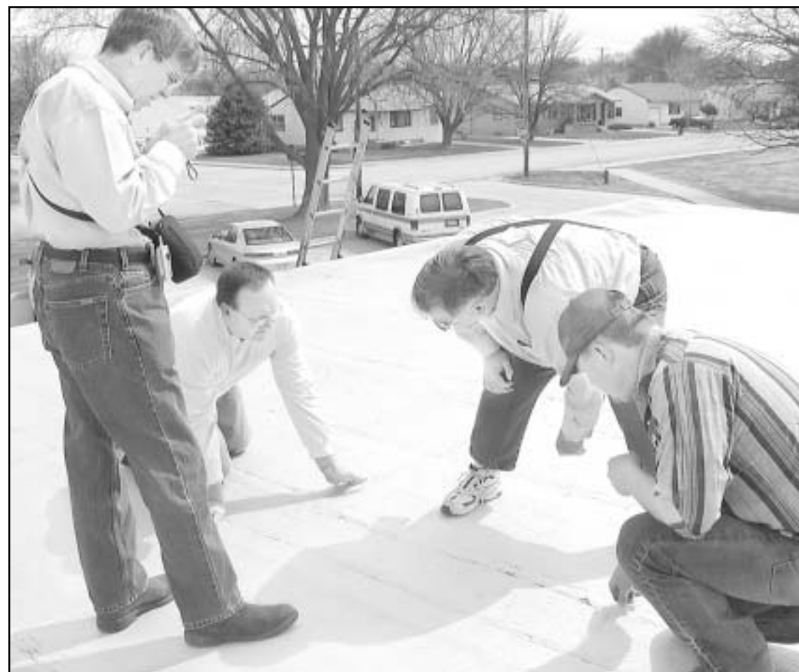
Norton Superintendent of Schools Greg Mann took pictures while school board members Jeff Nielsen and Chris Harding and roof consultant Joe Baker check out the roof of Eisenhower Elementary School. — Telegram photo by Veronica Monier
