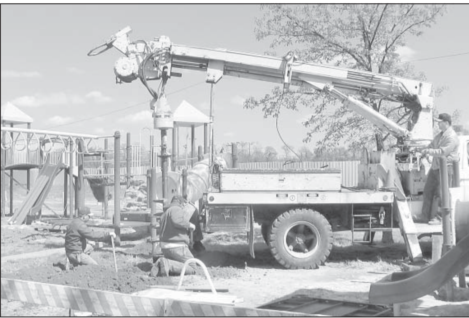
The new playground equipment at Elmwood Park is almost assembled. But, to get it done, a few more holes have to be drilled. Ed Lively (above) manned the drill yes-
