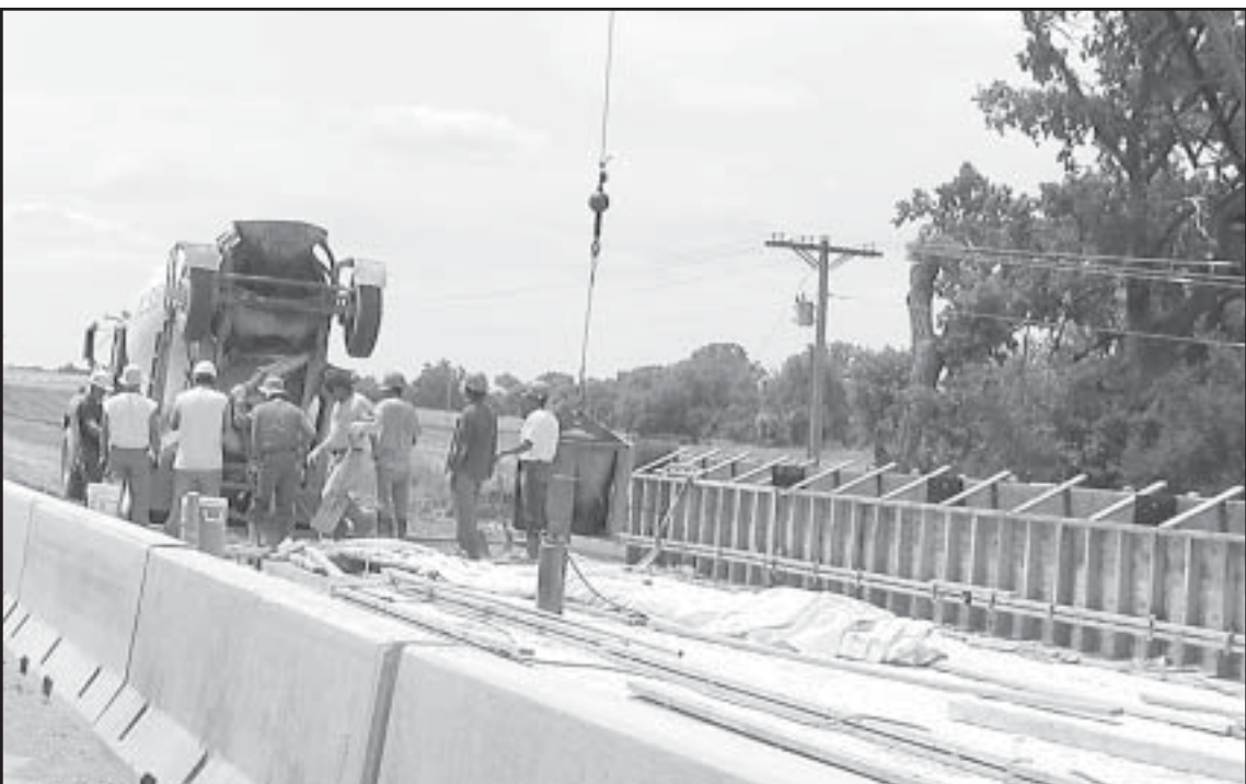
Construction crews will soon be done with the north half of the bridge west of Norton on U.S. 36. Once work is started on the south side, traffic will be moved to the north side. — Telegram photo by Carolyn Plotts
