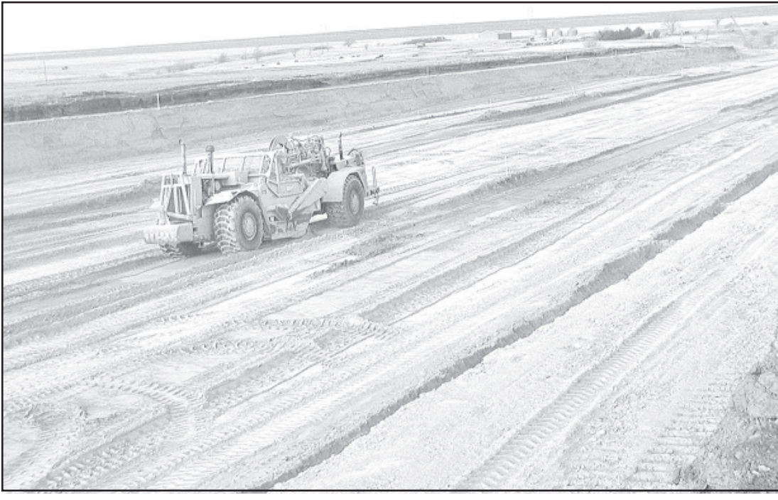
Mild winter weather has allowed road construction on US Highway 36, west of Norton to progress rapidly. An earth mover barreled down a wide piece of road just one mile east of Norcat. — Telegram photo by Carolyn Plotts
