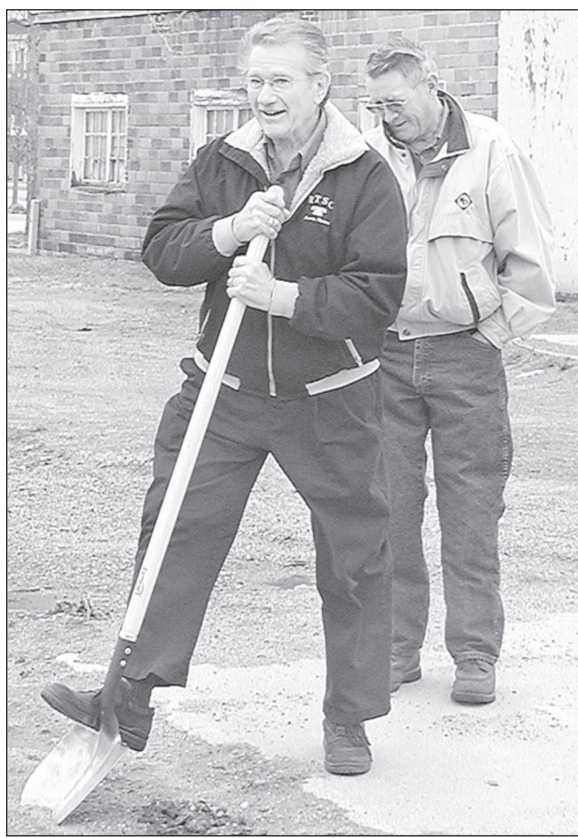
Rural Telephone's Larry Sevier made his mark at the groundbreaking ceremony for the Lenora Community Building last Friday, while Lenora Mayor Raymond Heikes, who had already shoveled his dirt, watched. — Telegram photo by Veronica Monier
