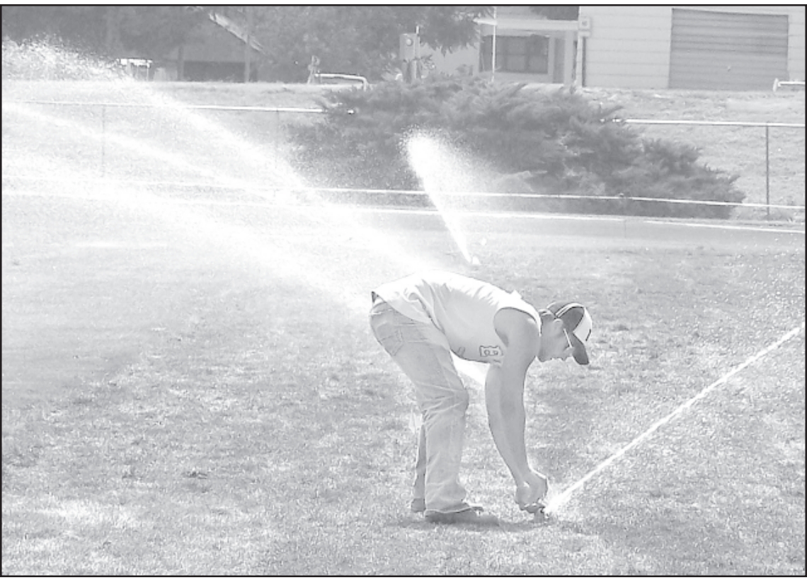
Kevin Lentz, an employee of Windmill Farms, adjusted some of the new sprinkler heads that were installed as part of the project. — Photo by Greg Mann
