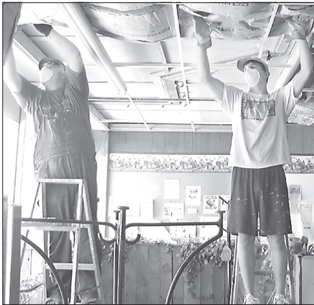
Friends of Jim Rowh, owner of Pure Prairie Natural Foods, poured in to lend a hand after the July 24 fire left his store with mild smoke damage. Some volunteers replaced new insulation and ceiling tiles (above) while others washed down the walls.
