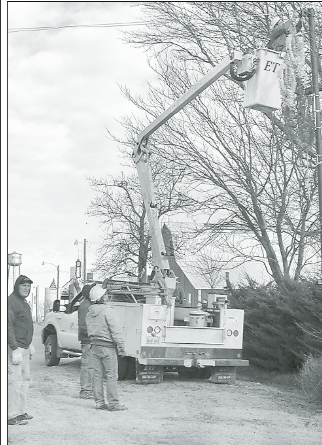
Linemen from Prairie Land Electric helped volunteers install Christmas decorations on Main Street in Norcat. — Telegram photo by Carolyn Plotts
