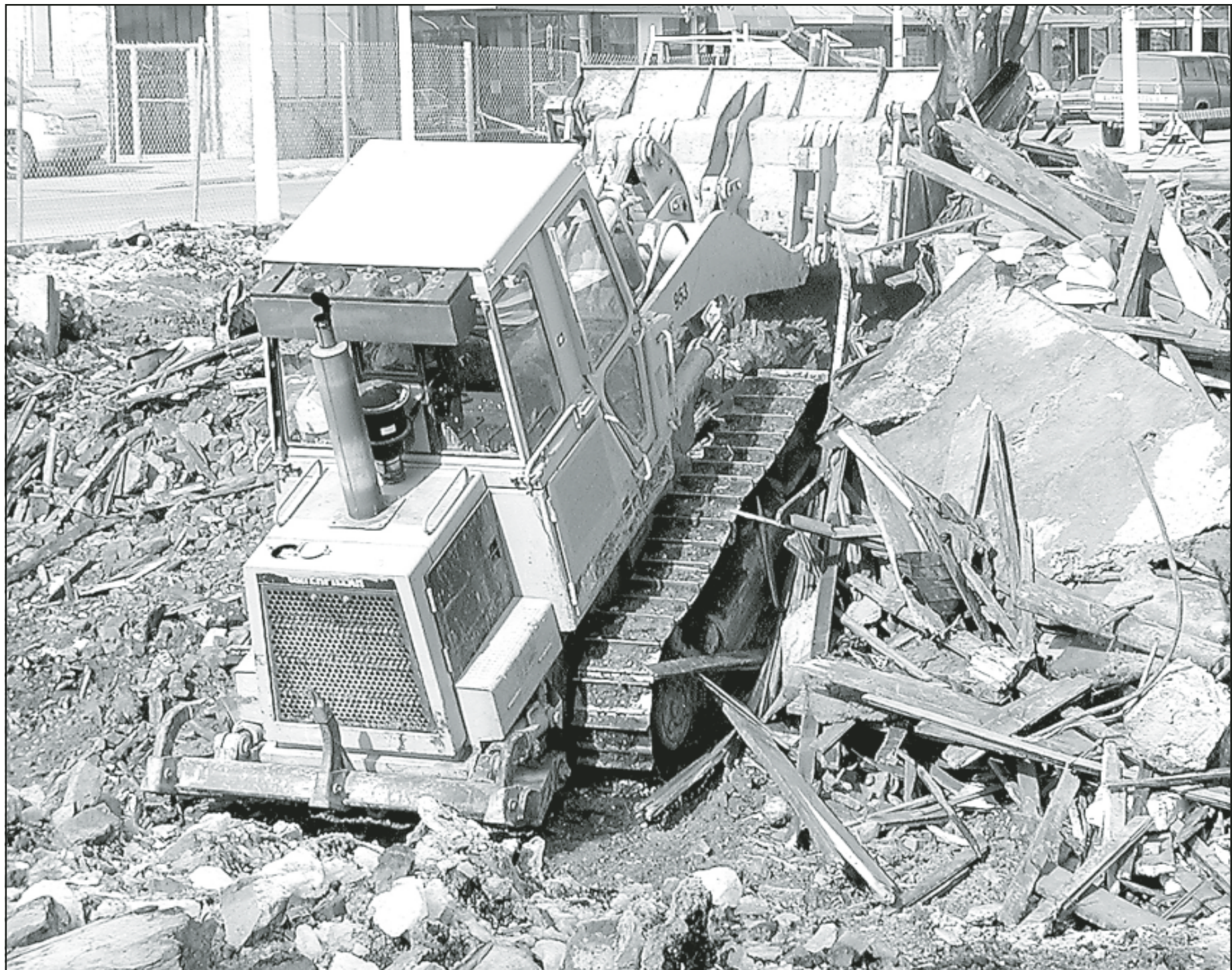
County and city crews began cleaning up the debris left from last fall's downtown fire Wednesday. By Thursday, almost all of the rubble was gone, leaving the hole ready to be filled with sand and dirt. — Telegram photo by Veronica Monier
