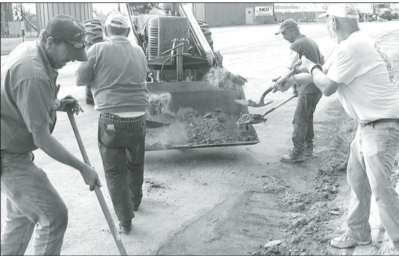
A crew of volunteers (above) scooped dirt from the gutters on Main Street to get downtown Norcatur ready for Memorial weekend. They were from left to right, Carl Lyon, Gary
