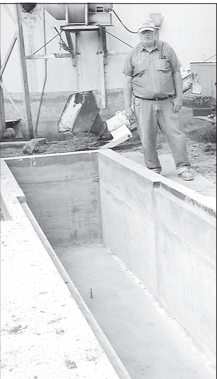
The new dump pit at Ag Valley Co-op is waiting for the auger to complete the project. Elevator operator Les Schievelbein stood by the pit that will make grain dumping much easier for truck drivers. — Telegram photo by Carolyn Plotts
