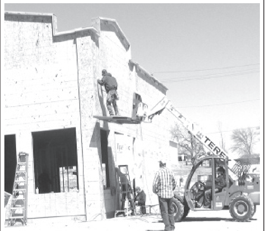
Progress on the new Subway Sandwich shop is evident to passersby on U.S. Highway 36. Last week there was just a concrete slab. By Monday walls were standing and it was wrapped with Tyvek housewrap. The national chain eatery is slated to open later this spring.
