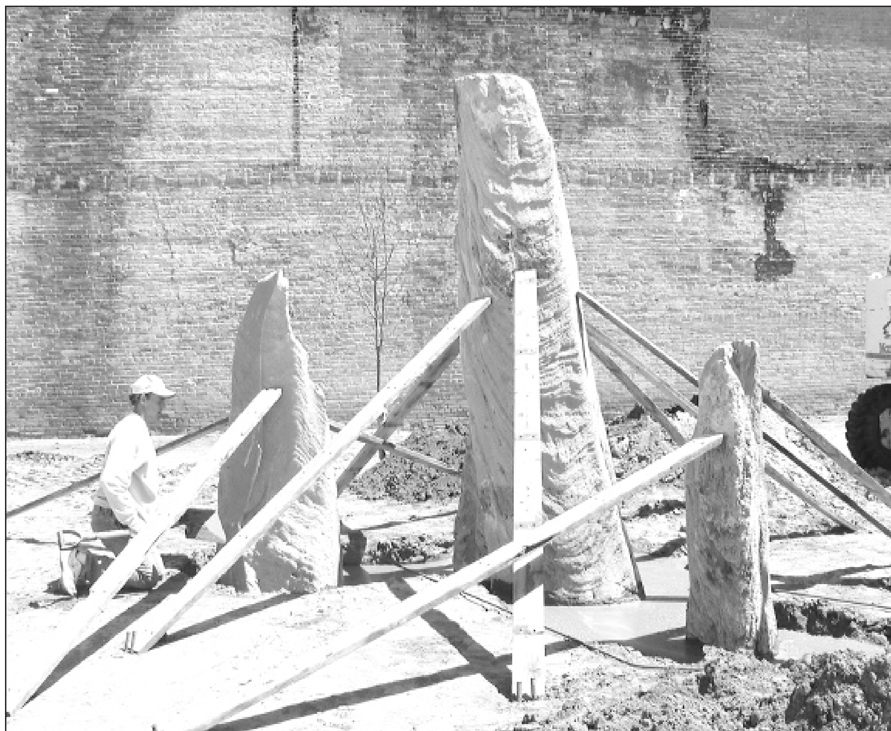
Stone pillars in Norton's downtown city park were installed Monday in a bed of concrete. They were braced with wooden supports until the concrete is completely set. Kirk Griffith was one of the installers. — Telegram photo by Carolyn Plotts
