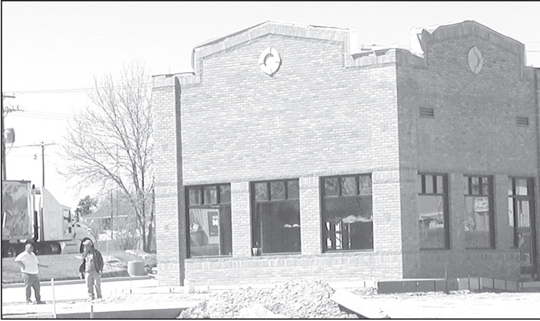
Brick masons are practically done with the exterior work at the new Subway sandwich shop on U.S. Highway 36 in Norton. The national sandwich franchise is scheduled to open later this spring.
