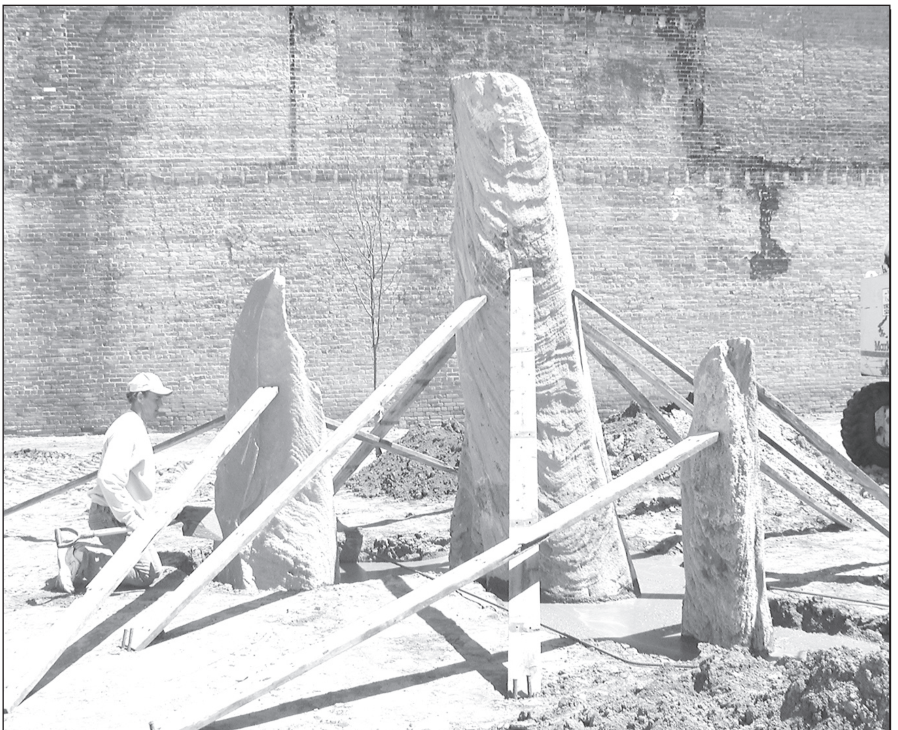
Stone pillars in Norton's downtown city park were installed Monday in a bed of concrete. They were braced with wooden supports until the concrete is completely set. Kirk Griffith was one of the installers.
