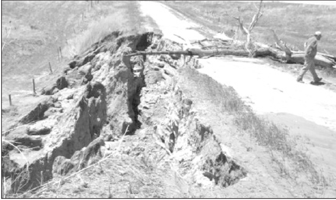
Topper Cook of the Norton County Road and Bridge crew inspected a huge wash-out on W-11 and Road N that happened last week during heavy rains. This was just one of the dozens of Norton County roads damaged by flooding.
