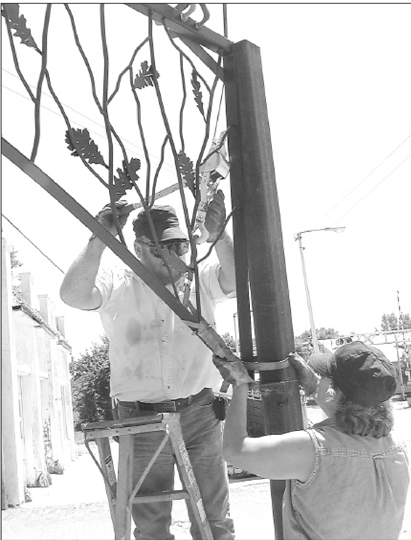
Metal artist Roger Fuller and his wife, Linda, used come-a-longs to winch into place the side panels of one of two pergolas in the new downtown park. Mr. Fuller spent the last month working on the panels in his Rawhide Ironworks shop. Mrs. Fuller designed the vine-like panels working with the Downtown Development Committee. The Fullers will complete the project by placing 2-inch by 10-inch redwood planks on edge to create the top of the pergolas.
