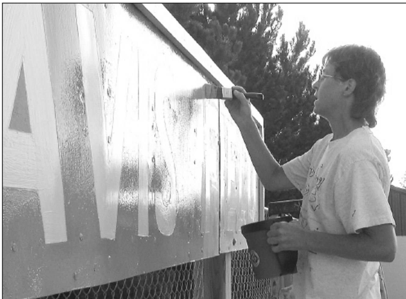
Kelly Lyon renews the paint on the Travis Field sign Thursday morning while the weather was cool.
