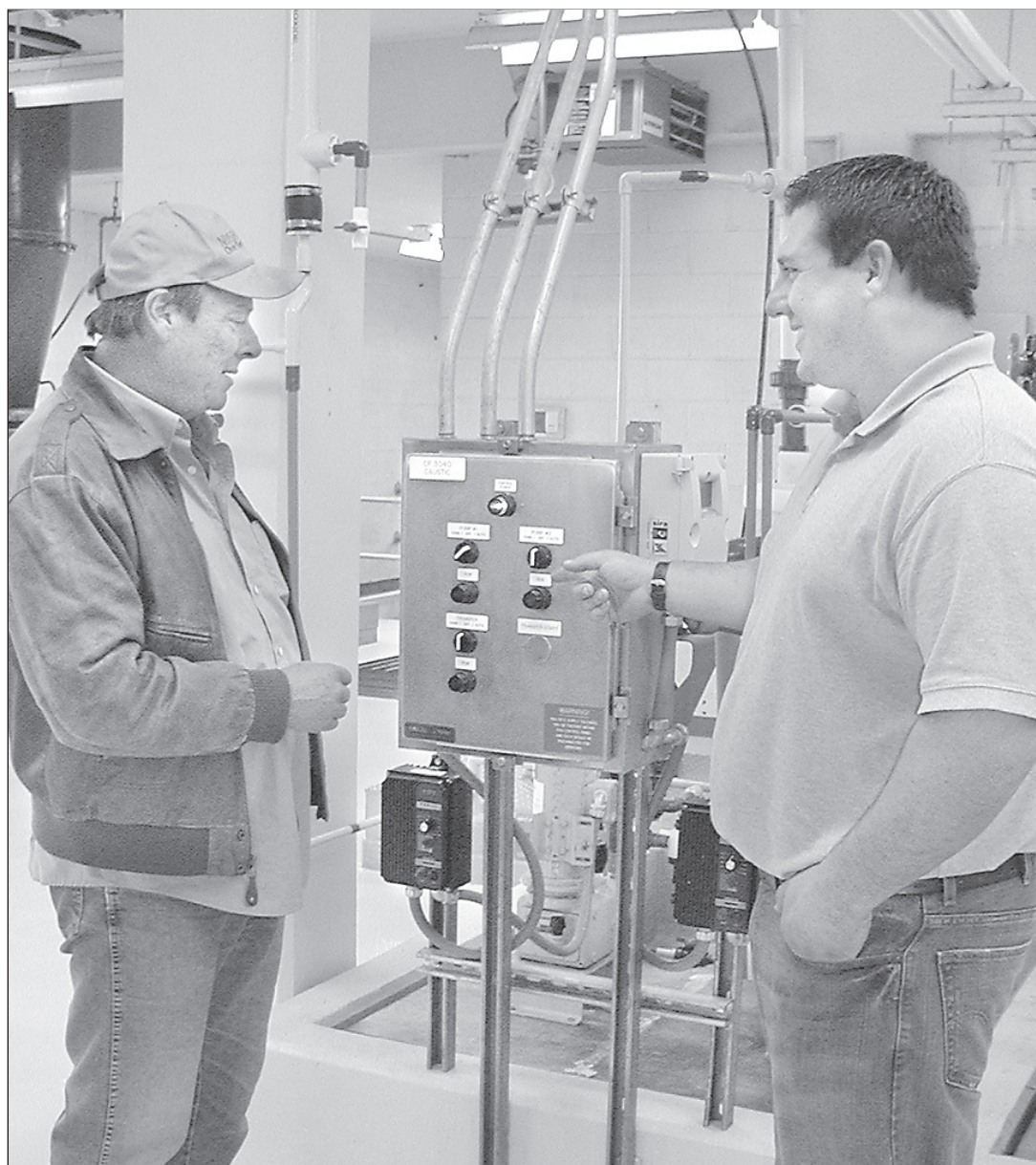
Chris Frack, Assistant Supervisor at the Norton Water Treatment Plant, gave his father, Jim Frack, a tour Friday afternoon during the open house.
