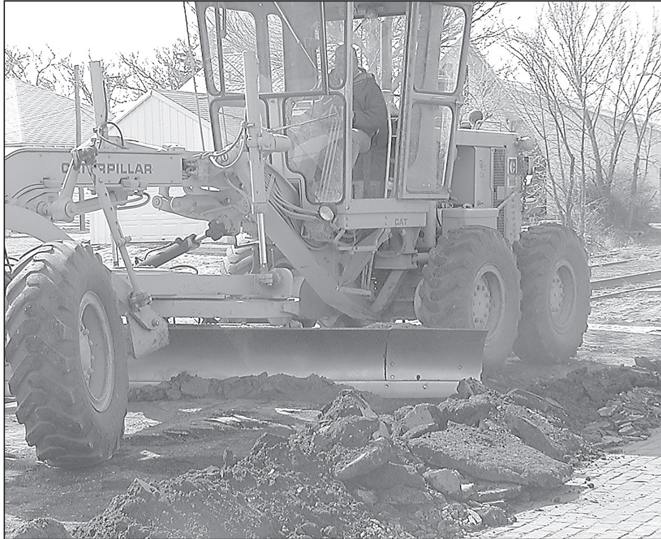
City employee Steve Reedy used a road grader to try to level out the asphalt on South Kansas Avenue at the railroad tracks Wednesday afternoon. Some of the leftover asphalt was used to fill in potholes on the other side of the tracks.
