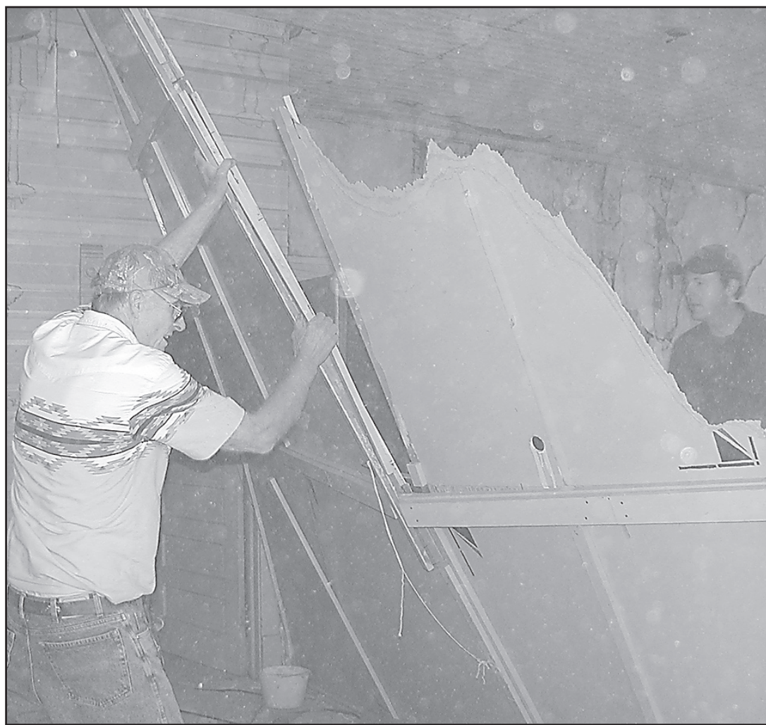
Norton County Commission Chairman Richard Thompson, left, and his son, Brian, tore down a wall in the Heaton Building Saturday morning. The building was donated to the Norton County Community Foundation, and will hopefully be turned into apartments once it is remodeled.
