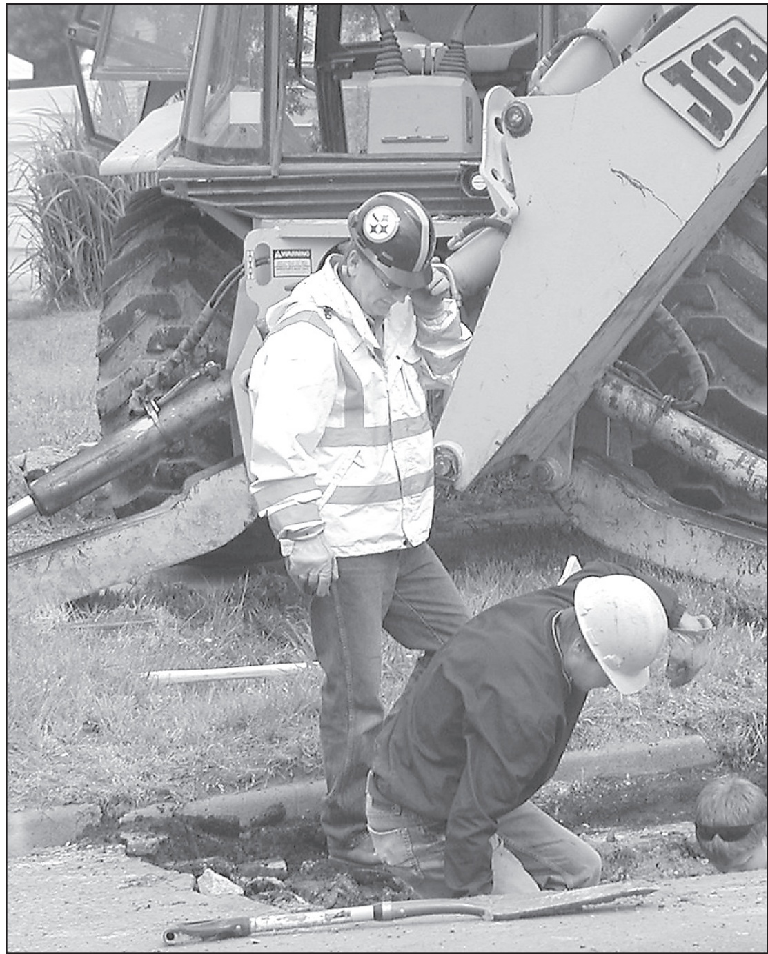
Norton public works supervisor Dan Bainter checked on Andrew Black and Bryce Engelbert who were repairing a water line on North State Street last Thursday.
