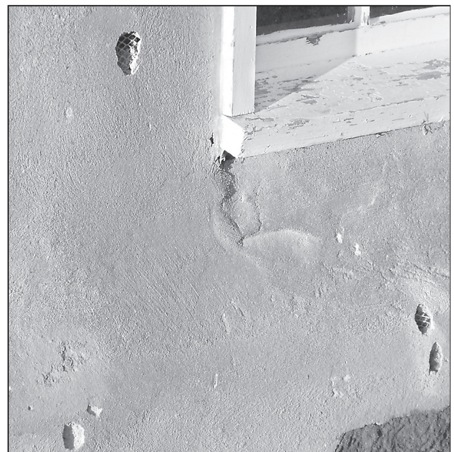
The Adobe House at Prairie Dog State Park was one of many buildings damaged during Friday's storm. Hail put dents in the wall and damaged the roof. Hail also damaged 40 camping units.
