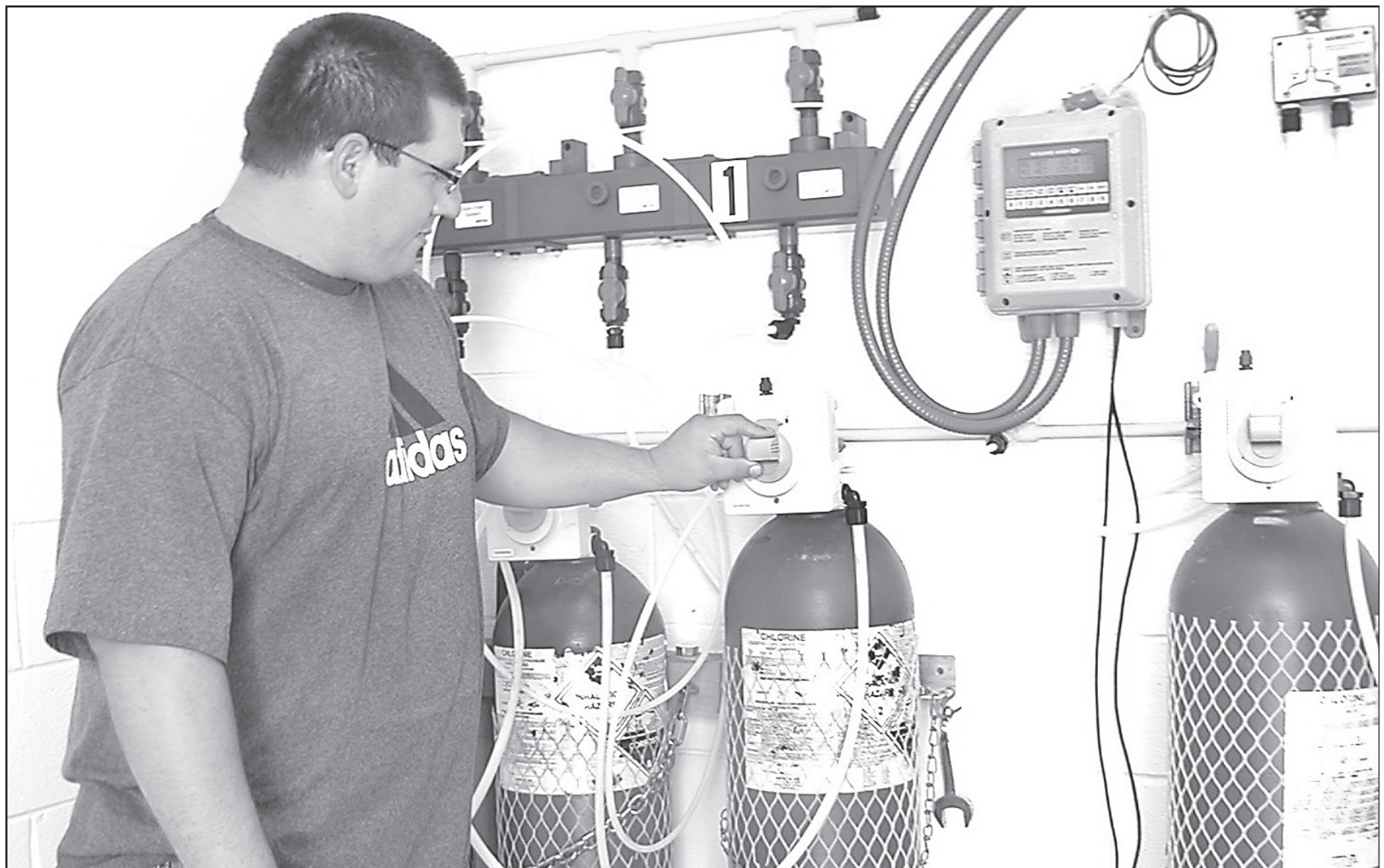
Water Plant Supervisor Chris Frack demonstrated the chlorine room at the Norton city water treatment plant on Wednesday. The chemical building was constructed when the city was forced to make upgrades
