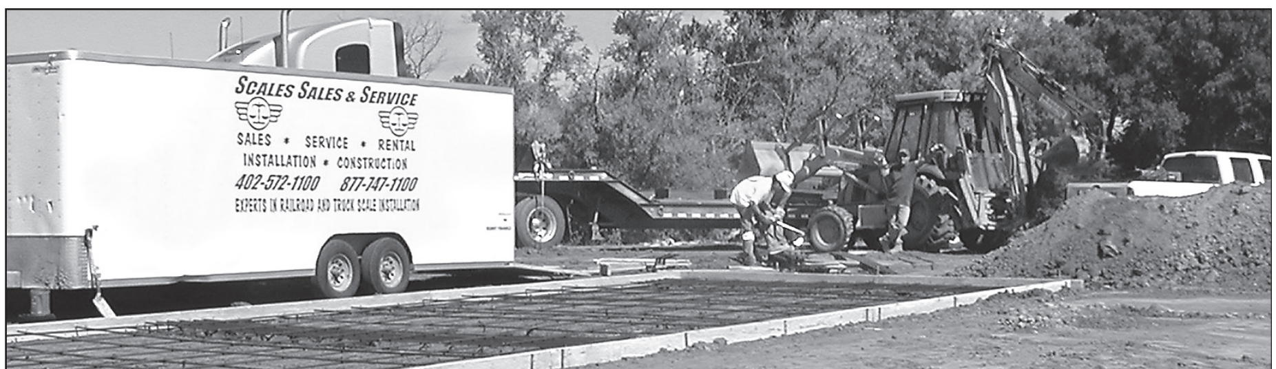
The new Ag Valley site is currently under construction two miles east of town, on Highway 36 and Road E2. The new site will house scales and pads and is expected to be completed by the end of September.
