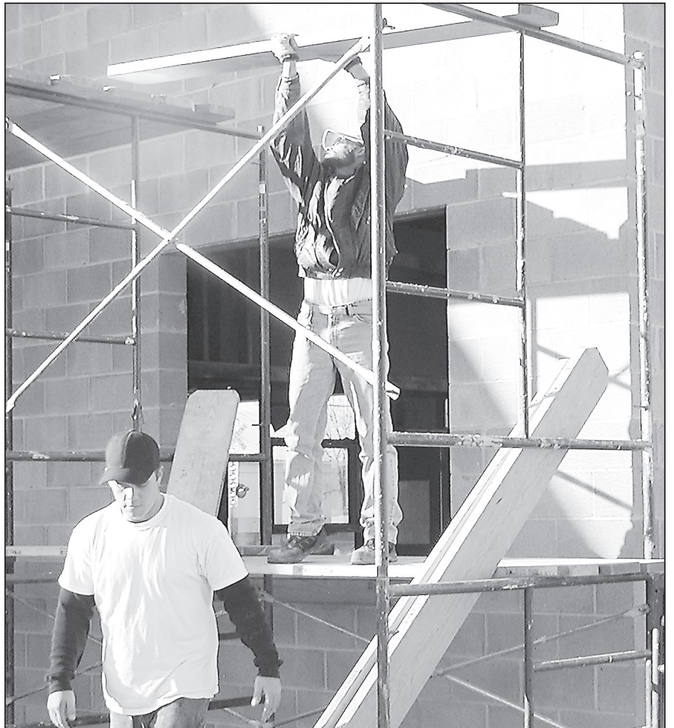
Work on the Moffet building began again this week with Paul-Wertenberger Construction starting the stucco work so Norton Glass Company could begin sizing windows. Interior work can begin as soon as the outside work is completed.
