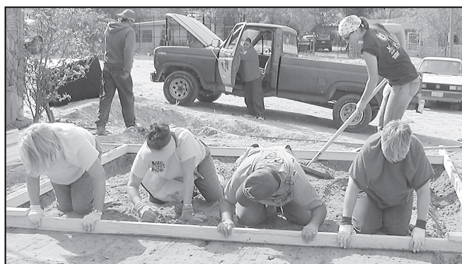
Mission team members from Norton, Oberlin and Norcatar worked to level the building site before the concrete foundation could be poured for the house they were building for a Mexican family.
