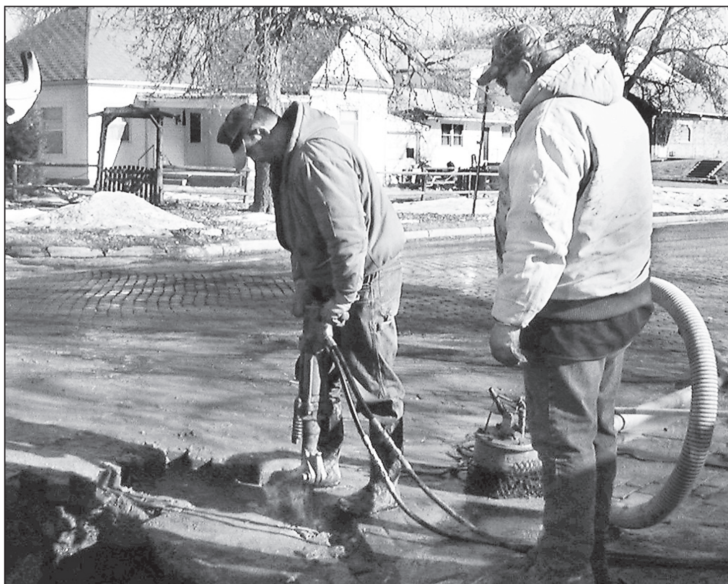
The public works crew was called to a water leak at E. Washington and Wabash Street on Wednesday. Public Works Supervisor Dan Bainter said he expected more water leaks
