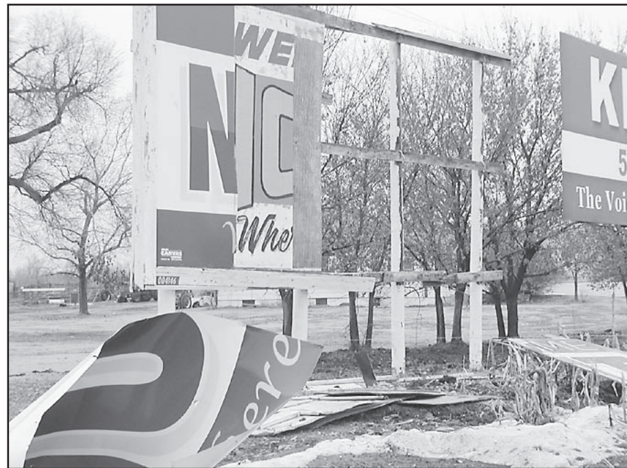
The Welcome to Norton sign on east Highway 36 was damaged during a recent storm. The sign does not belong to the city and sits on private property.
