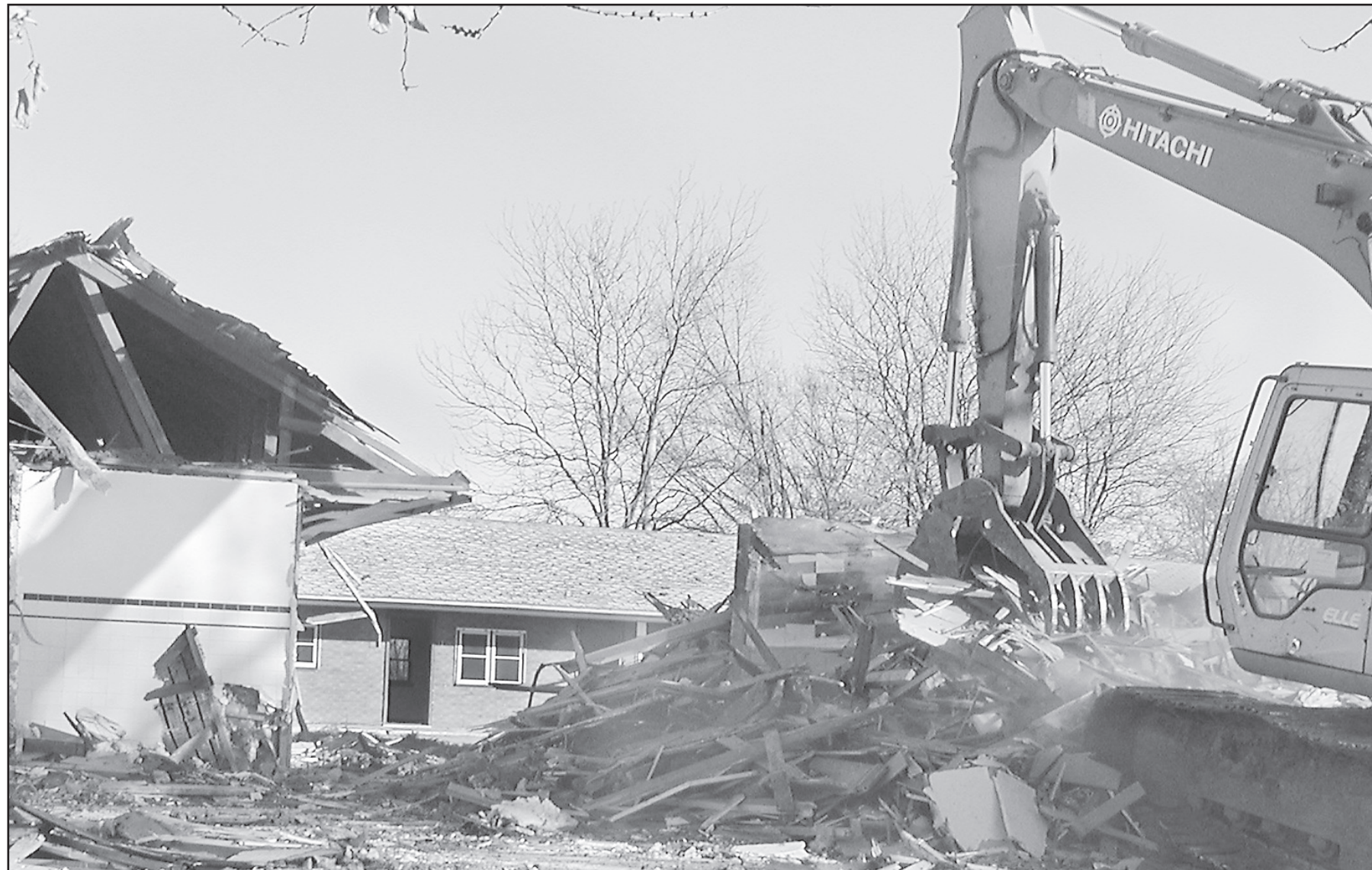
Whitney Construction started demolishing R&M Motel, located at 309 W. Holme. The site is expected to be the new location of Dollar General when they move to the highway. Bob Millan owned the hotel until he
