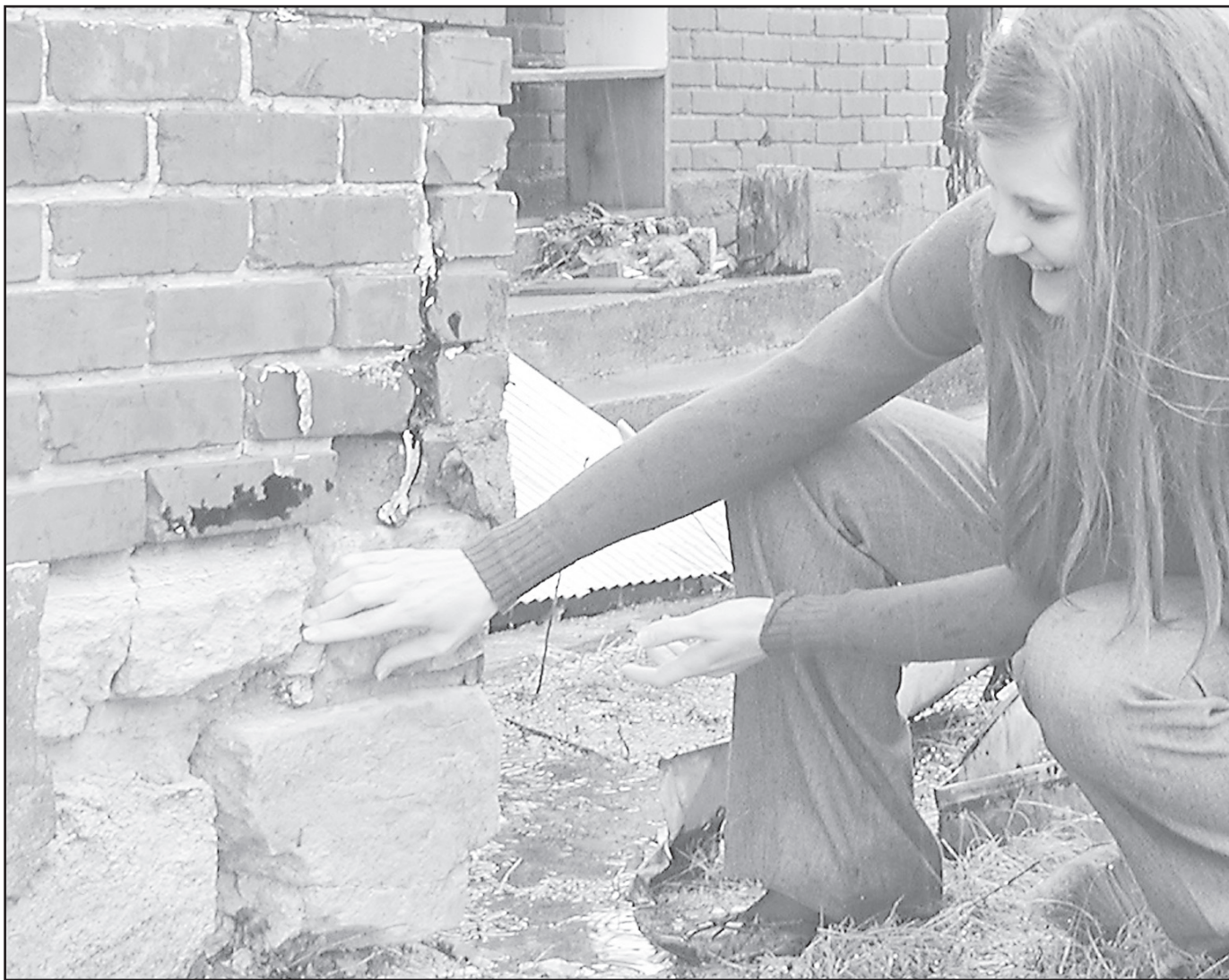
Norton City/County Economic Development Director Diane Stiles demonstrated the problems with the foundation at the Dr. E.A. Lyons House. Stiles received a $90,000 grant from the Kansas Historical Society, which will go towards fixing the foundation, roof, porch and brick.
