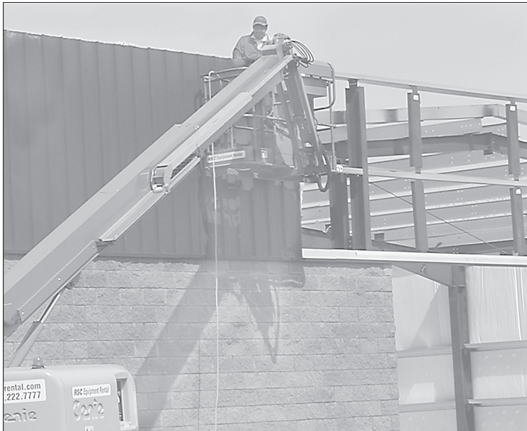
Construction of the new Dollar General store is moving quickly with the framework going up this week. The new store will be located on east Highway 36. It is not yet known when construction will be complete. Whitney Construction was hired as the contractor. —Telegram photo by Erica Bradley
