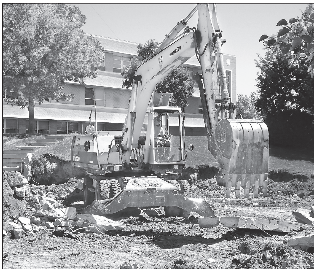
Clearing of the property just south of the Norton County Hospital began this week in order to prepare for the building of the new Norton Doctors Clinic. Courtesy photo
