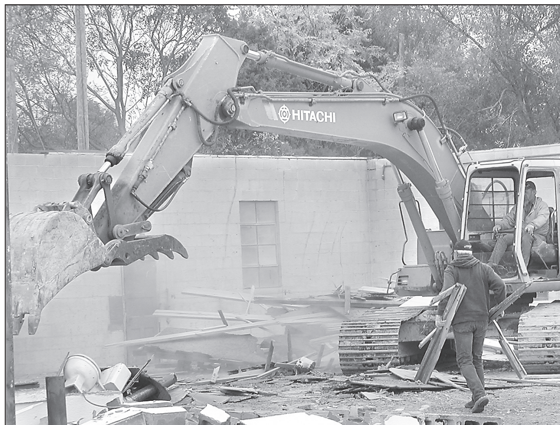
A crew working for Whitney Construction and Farms Inc. brought in heavy equipment Monday to demolish the former Kansasland Tire building. The property is being cleared to make way for a new hotel.
