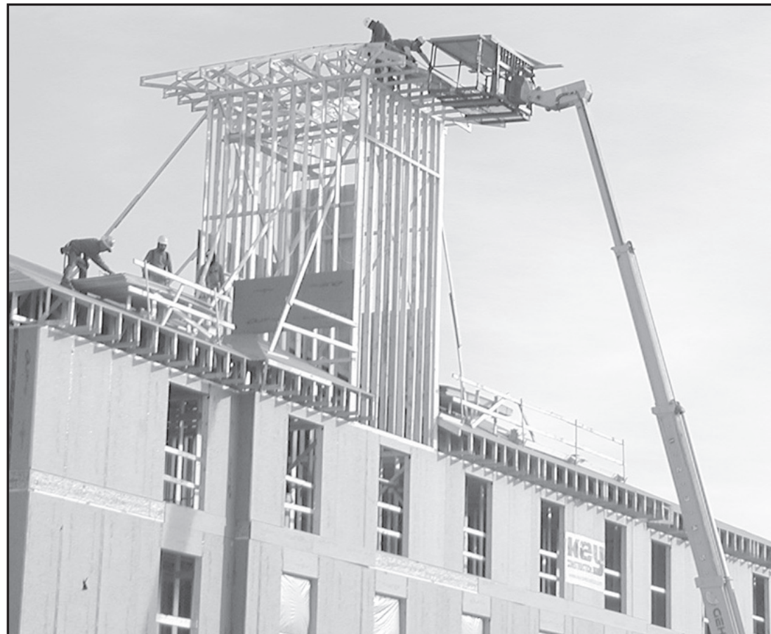
The completion of the new Sleep Inn Motel on U.S. Highway 36 is getting closer. On Wednesday, a crane lifted the roof panels up to the workers who had already climbed the tower.
