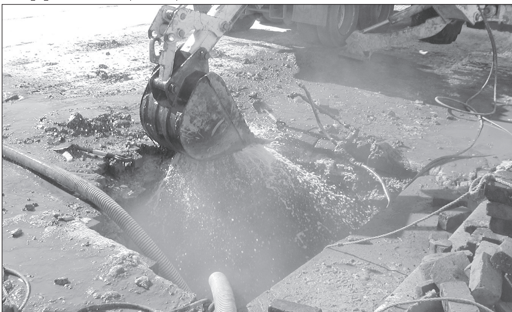
The bucket on the back hoe puts a lid on the water break that occurred on Wednesday in front of First Security Bank. Dan Bainter, Public Works Supervisor, said "The pipe that broke was an old galvanized pipe that had outlived its usefulness. Most of the pipes that are breaking now are pipes that were put in when the city was built, they were not made to last this long." -Telegram photo by Harriett Gill
