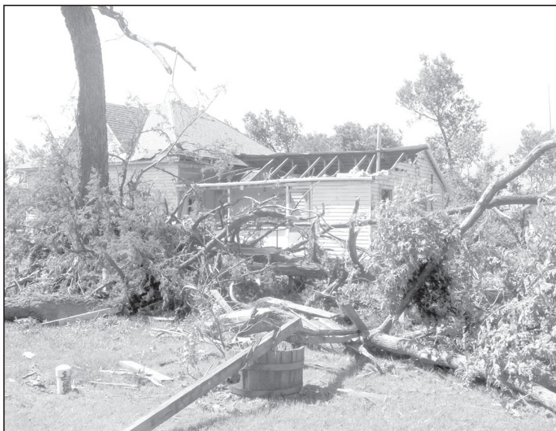
This home just northeast of Alma was heavily damaged by a severe storm and tornadoes that swept through the area early Monday afternoon. -Telegram photo by Carleen Bell
