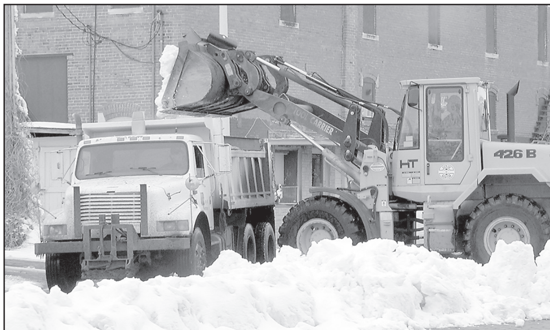
After about 8 inches of snow fell across the area over the weekend, Norton city crews spent the week clearing the snow that had been plowed to the middle of the streets in town. The snow is loaded into dump trucks and taken to a city lot just south of Elmwood Park where it is left to melt. Pictured, street crews cleared a portion of South Kansas Avenue Tuesday afternoon on their route through town.
