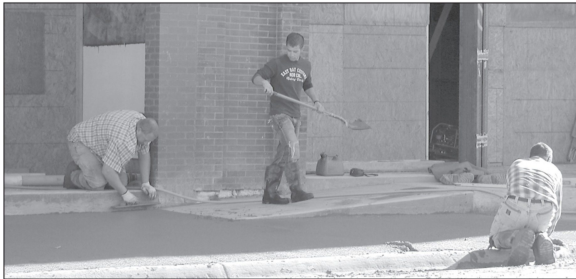
The last bit of concrete was poured on the west side of the Heaton Building in Norton on Tuesday. Cornerstone employees, Kallen Saun-
